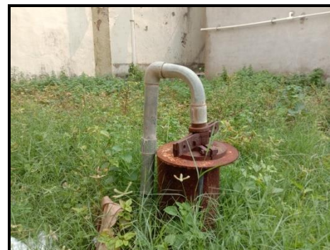
Figure 3. Bore well system in the college campus
